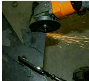
Guard missing on grinder
