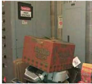
Housekeeping issue in electrical room
