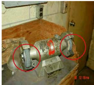
Guards missing on bench grinder
