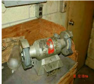
Grinder is not mounted to bench top
