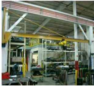
Load limit on jib crane is not visible
