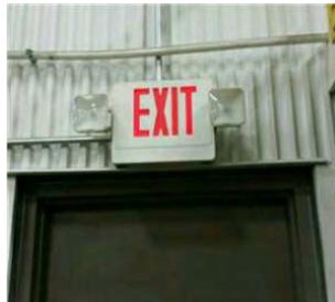
Emergency lights not working above east door in warehouse
