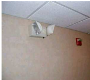
Emergency lights not working when test button is depressed
