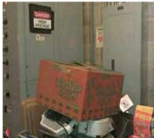
Blocked electrical panels
